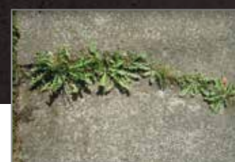
Weeds on pavement
