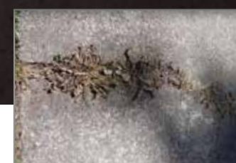
Weeds on pavement 2 - 5 days after treatment
